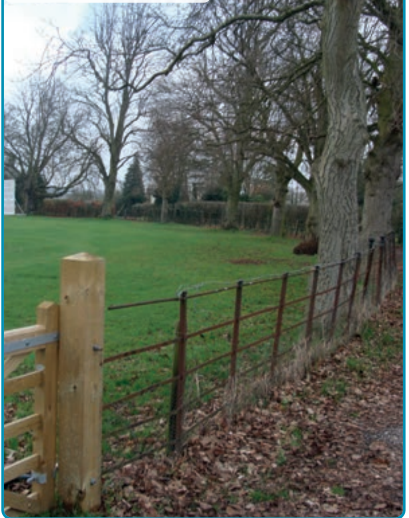
Picture 5 – Cricket Ground, quintessentially English. Railings are in need of repair.
