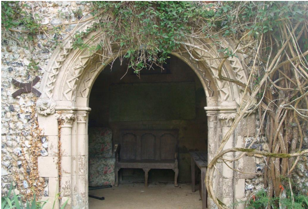
Picture 8. Grade II summer House, a building included on the Council's Heritage at Risk Register.
