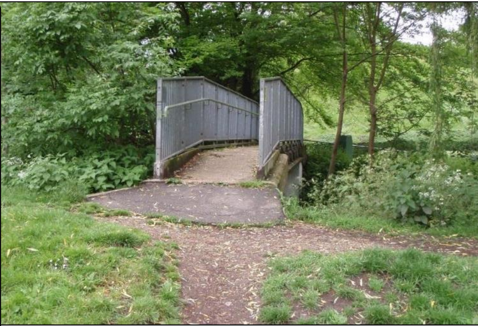
The previous bridge was narrow, poorly positioned and with no onward surfaced connection.
